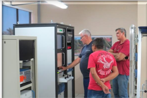
1: Power On and Tests Support
