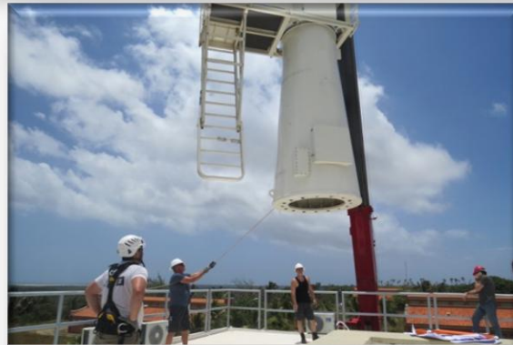
1: Pedestal Installation Support
